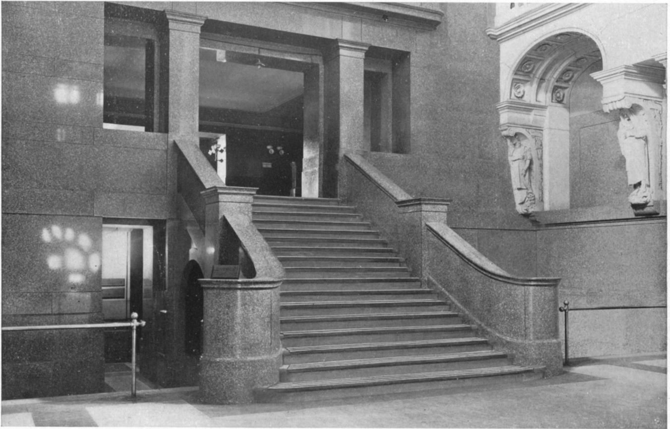
MASON SAFETY TREAD (STEEL AND CARBORUNDUM) Repairs on hard Italian Marble, Main Stairway, Suffolk County Court House, Pemberton Square, Boston, Mass.
