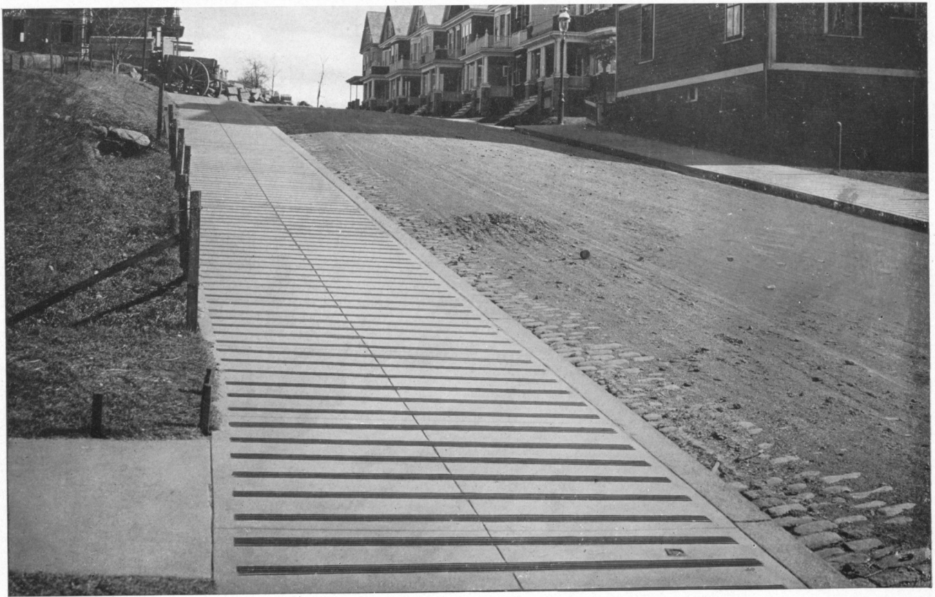
MASON SAFETY TREAD (STEEL AND CARBORUNDUM) ON INCLINED GRANOLITHIC SIDEWALK at Longfellow Street in Dorchester, a suburb of Boston, Mass.
